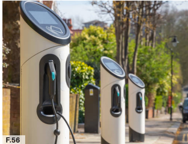
Figure 56: Examples of on-street car charging points.
