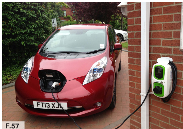
Figure 57: Examples of off-street mounted car charging points.
